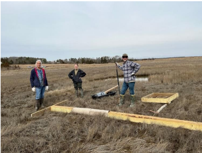
Dave Frederick, Taylor Schmidt and Ben Wurst (L to R) ready to install the platform!
